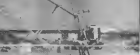
A spectacular sight for sidewalk engineers was the moving of the water tower near the Cobay Commissary. Three cranes and a tractor did the job. The whole tower was lifted into the air by the cranes and then lowered slowly while the tractor pulled it to a horizontal position. The tower will be moved to the Plant Commissary area.
